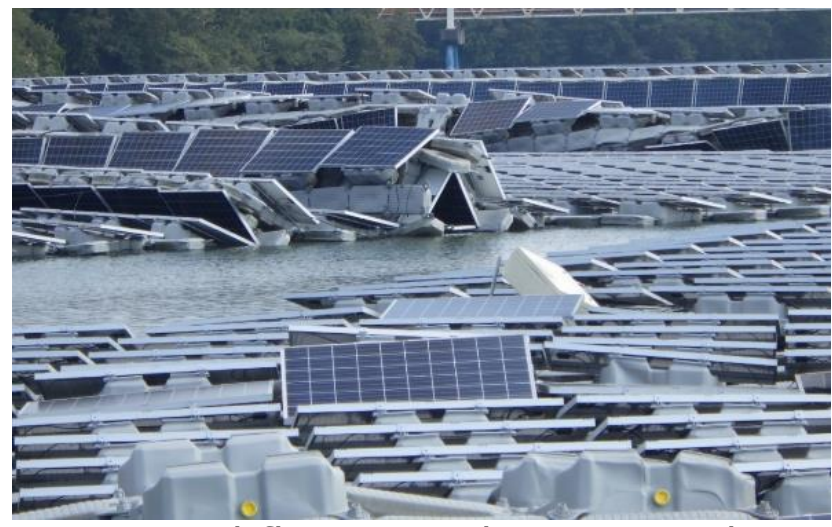
Damaged floating solar power plant
